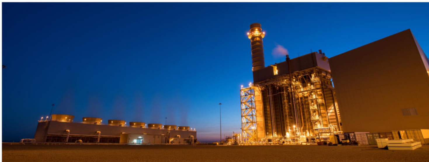
Carty Generating Station, our 440 MW natural gas baseload plant near Boardman, Ore.
